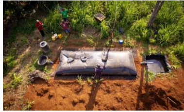
Sistema.bio digester in Gujarat, India
